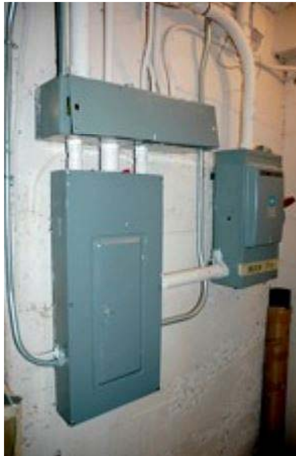
Main electrical panel in basement
