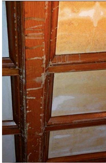
Damage from the fire
