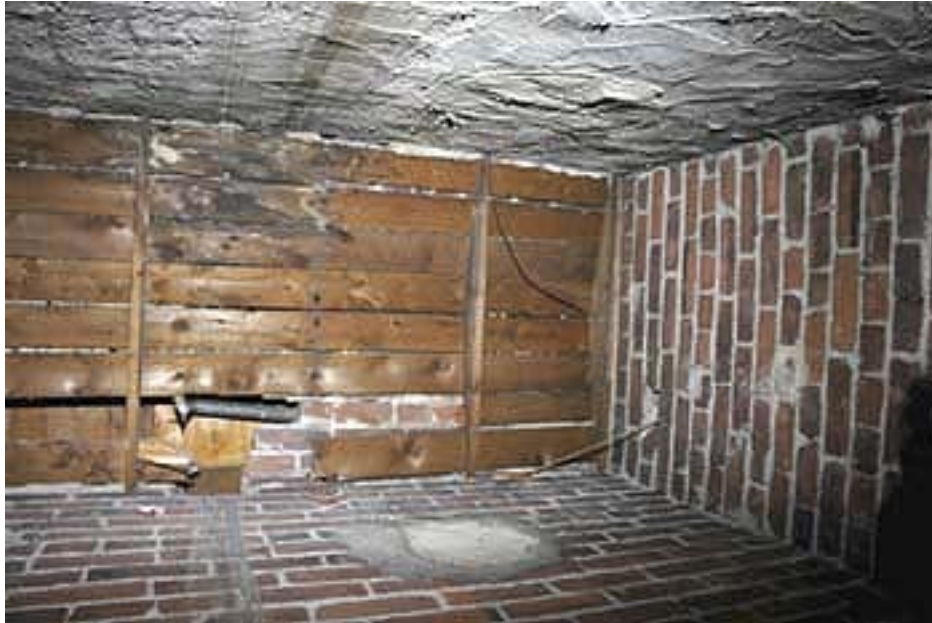
The area above the hole in the wall in the basement
