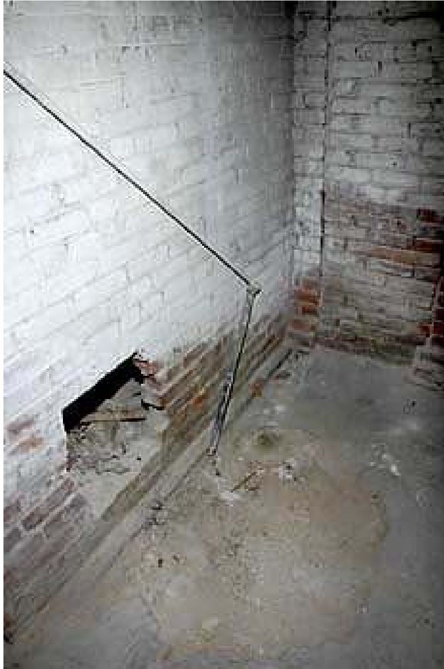
Hole in the wall and floor in the basement
