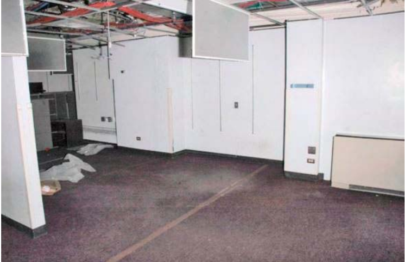
Library that had flooded
