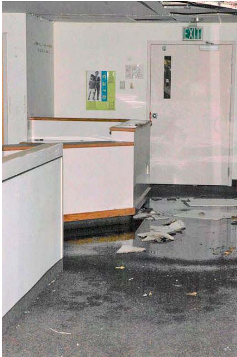
Flooding during the demolition
