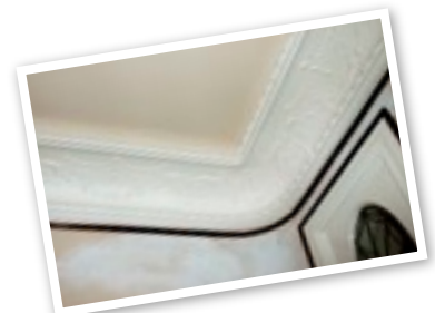
“imperfect” ceiling corner
